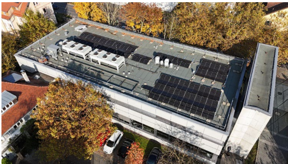
Figure 11: Part of the photovoltaic system, installed 2024 at the Zwingenberg site in Germany
